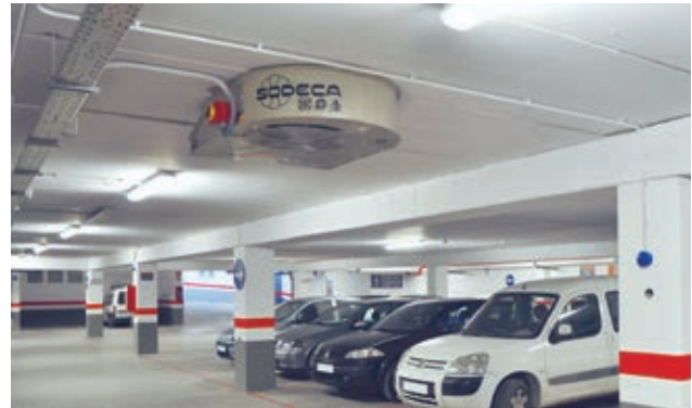
CI installed in a car park
