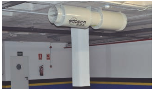
THT/IMP installed in a car park
