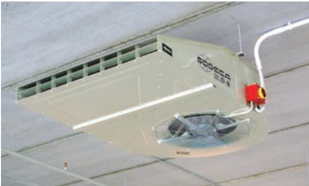
CI installed in a car park
