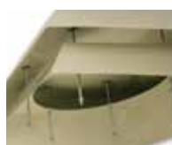
Hood with natural outlet air due to differential pressure
