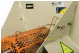
External grease fittings to make maintenance easier
